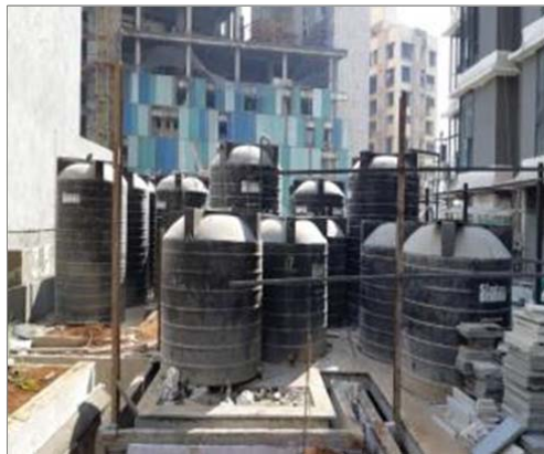
Drinking Water tank for Labor camp
