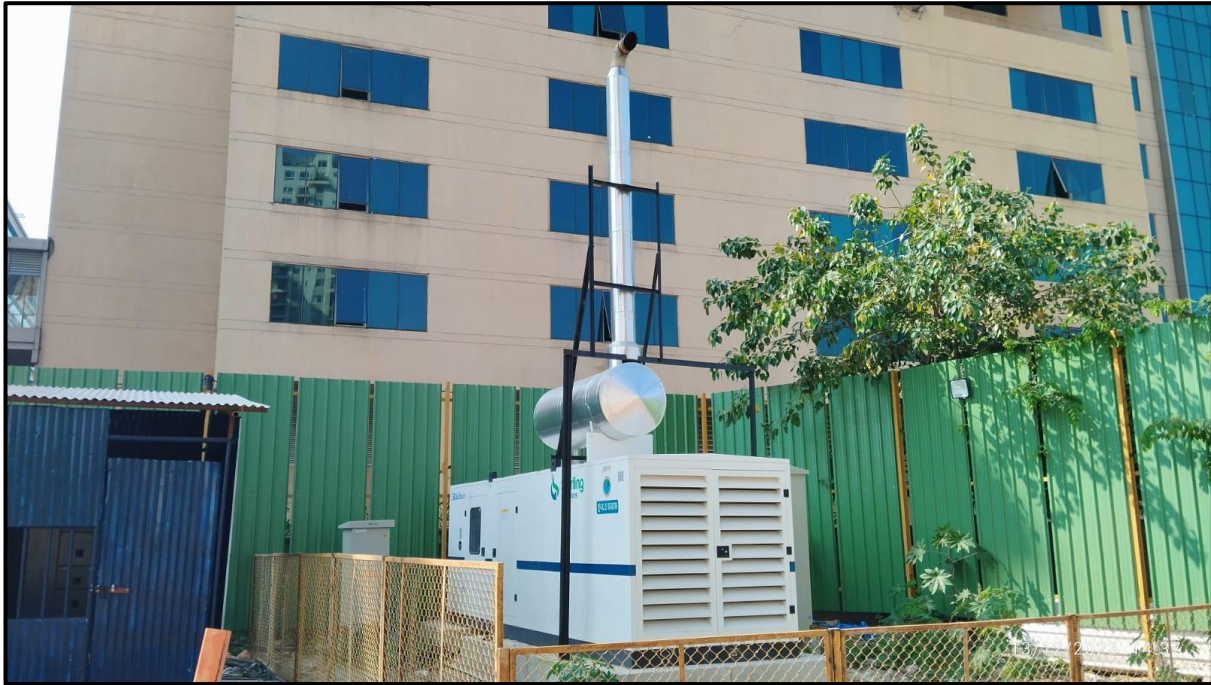
Photograph: Enclosed Type Silent DG Set
