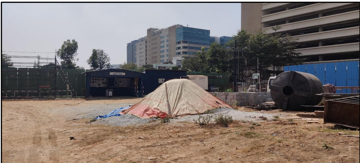
Photographs: Loose Construction Materials is Covered using tarpaulin sheets
